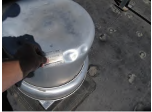
Figure 9: 1-1/2" diameter indentation in metal vent cover
