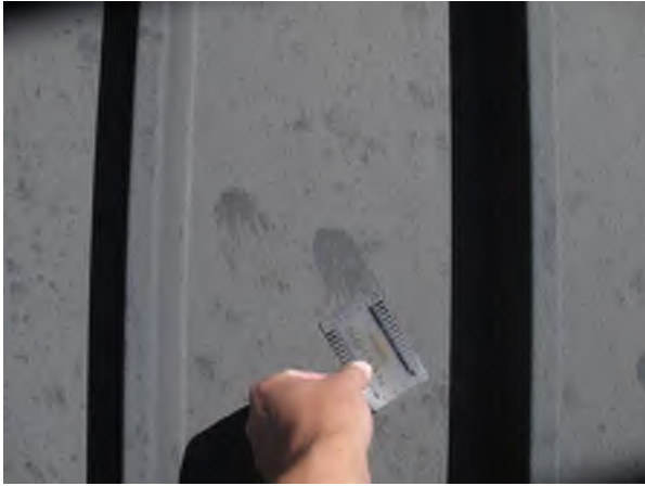
Figure 8: 1-1/2" burnish mark on south facing metal roof panels
