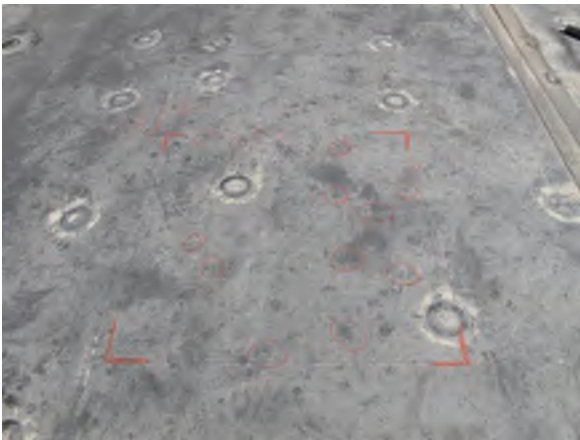
Figure 33: Overall view of 2'x2' sample area 1 on lower roof section of City Hall
