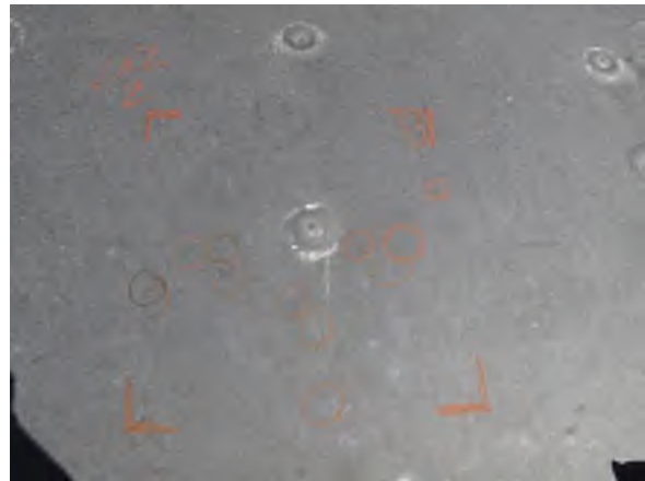
Figure 34: Overall view of 2'x2' sample area 2 on upper roof section of City Hall
