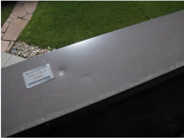
Figure 10: 1" diameter indentation in metal parapet coping
