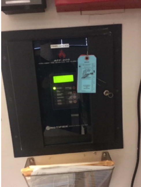
Existing Fire Alarm Panel
