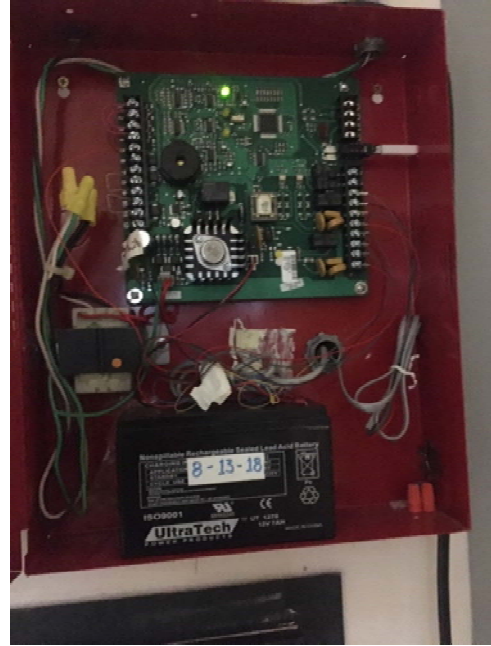
Existing Fire Alarm Panel
